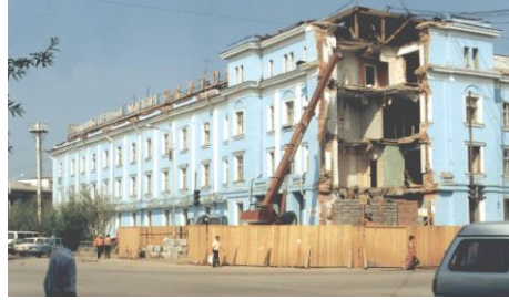
Figure 1. Destruction of the building in the centre of Yakutsk (Eastern Siberia), 1999.
